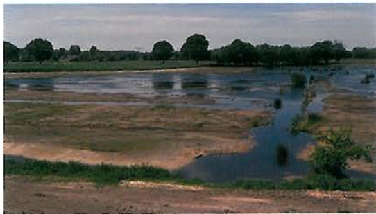
Figure 8.1 - Mosbulten (NL). Above: to compensate for the loss of marshland habitat due to the construction of Highway A50 Eindhoven-Oss, the first thing to do was transform set-aside farmland by removing the top soil. Below: after removal of the soil of former arable land, marshland habitat may develop and attract breeding birds. Target species are reed warbler and water rail. (Photos by H. Bekker)
