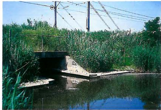
Figure 7.63 - An adapted culvert under a railway in the Netherlands. The ledge needs a good connection with the embankment, a width greater than 0.7 m and to be made of concrete, stone or wood. The design should be as open as possible. (Photo by H. Bekker)
