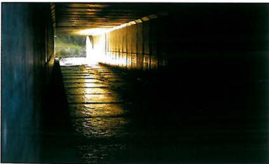
Figure 7.67 - Baffles in a fish passage in Norway during and after construction. (Photos by B. Iuell)
