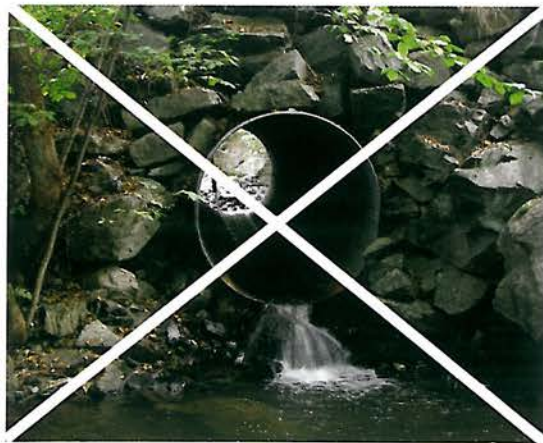
Figure 7.66 - This pipe in Norway was placed too high above the stream. The outfall drop creates a barrier to fish moving upstream. (Photo by B. Iuell)
