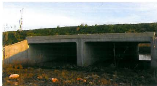
Figure 7.46 - This passage under a road which crosses a protected wetland in Spain (Natural Park Aiguamolls de l'Empordà) was constructed with a dividing wall to reduce costs: Dimensions of each section: 10 m wide (5 m each section), 2 m high, 28 m long. It is used by mammals, e.g. otter, polecat, badger and wild boar, but also by some birds from the adjacent wetland. (Photo by C. Rosell)
