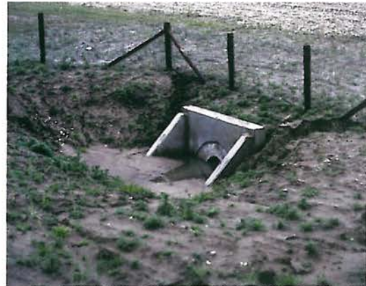
Figure 7.57 - This tunnel in the Netherlands has been filled with sand and water. The lesson learned from this example is to construct a tunnel above the ground water level and to build stable slopes around the entrances. (Photo by H. Bekker)
