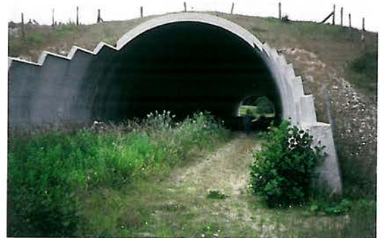
Figure 7.49 - This underpass in Denmark has a diameter of 13 m with 8 m clearance, and is 87.5 m long (at the top), 115 m (at the bottom). It is regularly used by fox, badger, marten, stoat and polecat - as well as by humans and horses. For ungulates the openness index would be too small. For underpasses under motorways the layer of soil above the overpass should be thicker to reduce noise inside the underpass. (Photo by B. Wandall)
