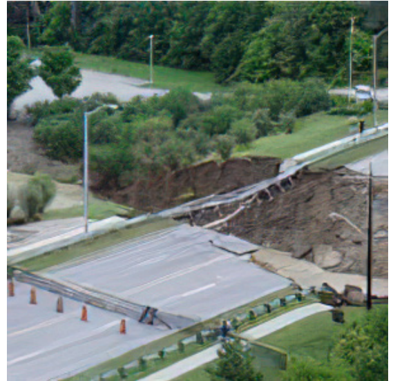
Washed-out culvert on Toronto's Finch Avenue.
